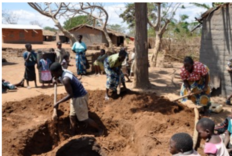
Figure 15: Photograph of both the community women and men contributing to the construction of the pilot project
